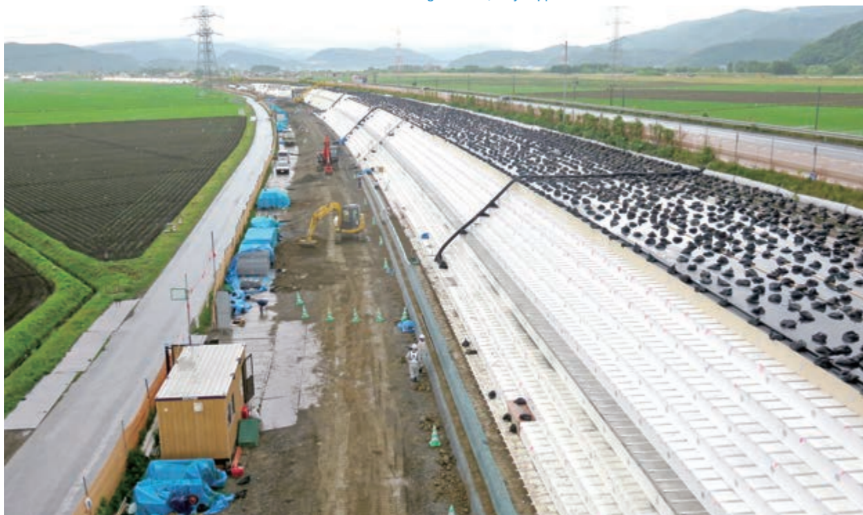
Soil Blocks work behind the scenes. Although unseen, they support roads and reclaimed land as embankment material
