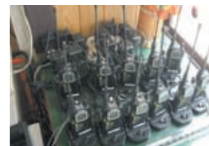
Disaster-prevention wireless equipment (Shiga Plant)
