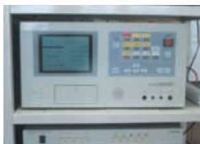
Emergency information transmission system (Shiga Plant)
