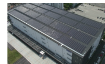
Photovoltaic power generation equipment installed at the Kaneka Takasago Distribution Center
