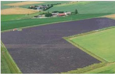
Large photovoltaic power system installed on a farm in Germany (photo courtesy of IBC Solar)
