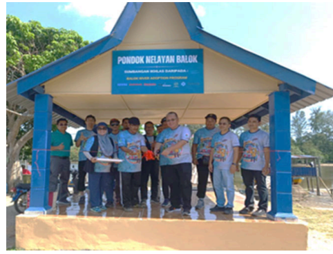
Building a community hut on the river pier (Kaneka (Malaysia) Sdn. Bhd.)
